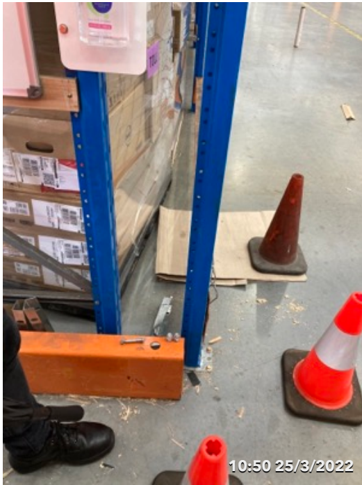
Photo 39 Property damage minor incident Evidence of reported to Manager refer to email.
