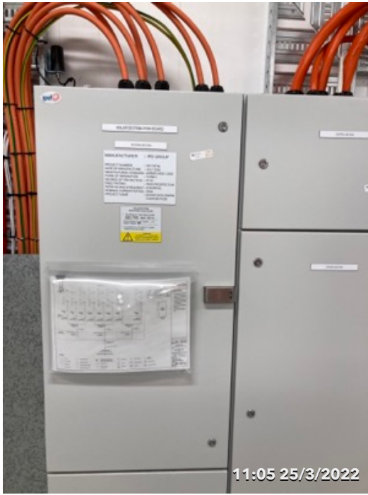
Photo 54 Solar Panel Distribution Board
