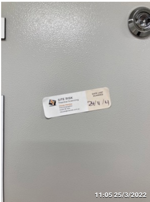
Photo 55 Test and tagged Solar Panel Distribution Board
