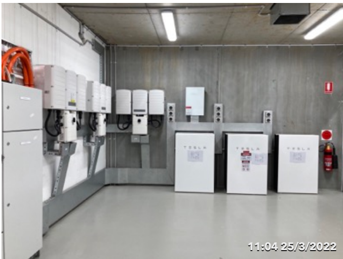
Photo 51 Solar panel batteries
