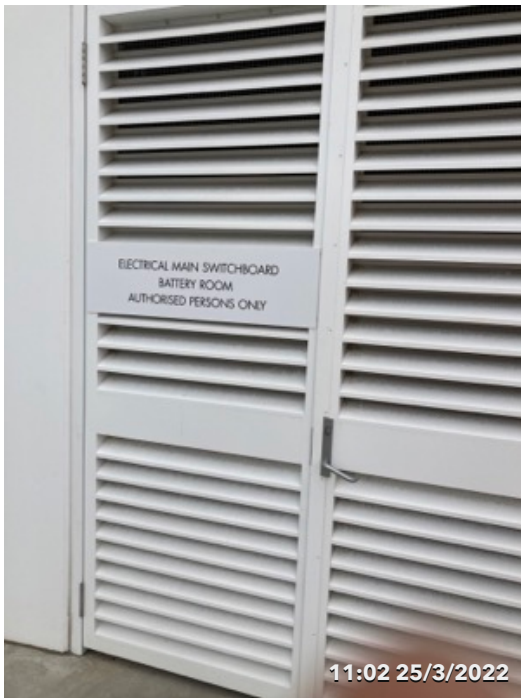
Photo 49 Electrical main switchboard
