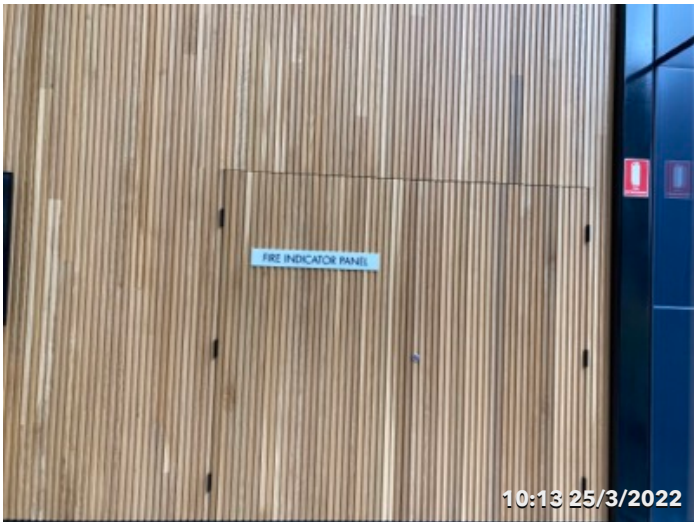
Photo 6 Fire Indicator Panel
