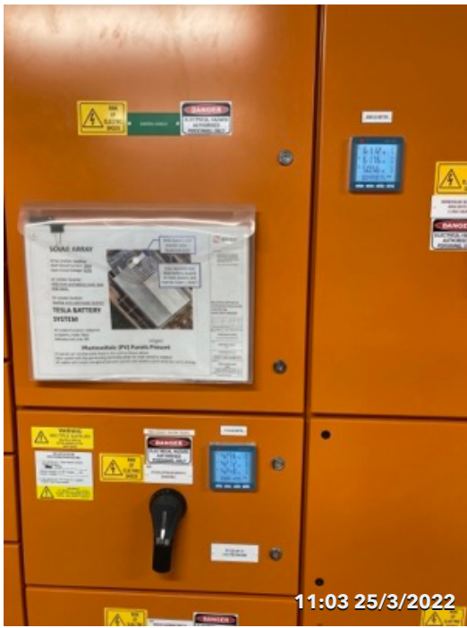
Photo 50 Electric main switchboard
