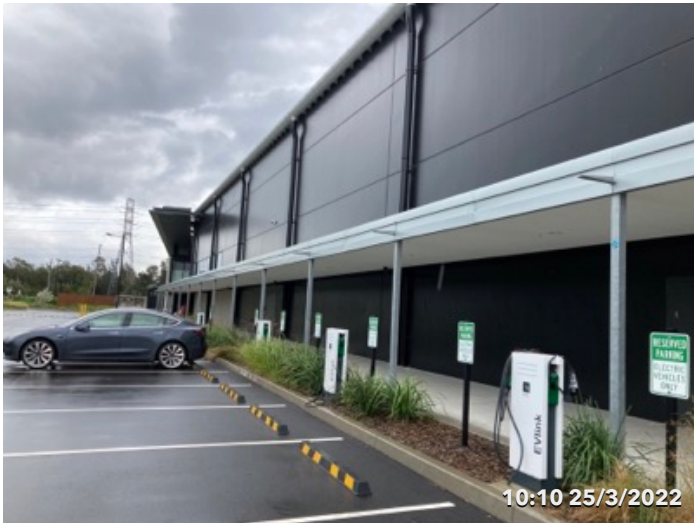
Photo 1 Electric car charge bays
