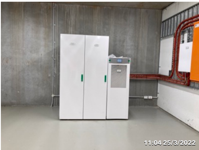
Photo 53 Back up power
