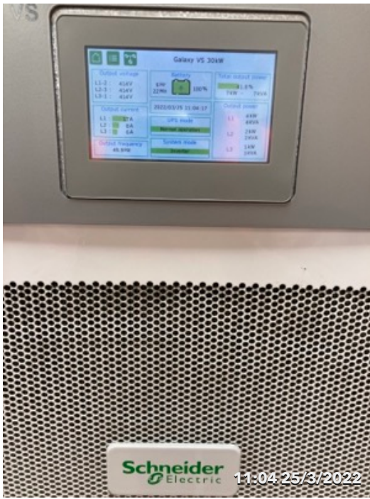
Photo 52 Emergency backup power
