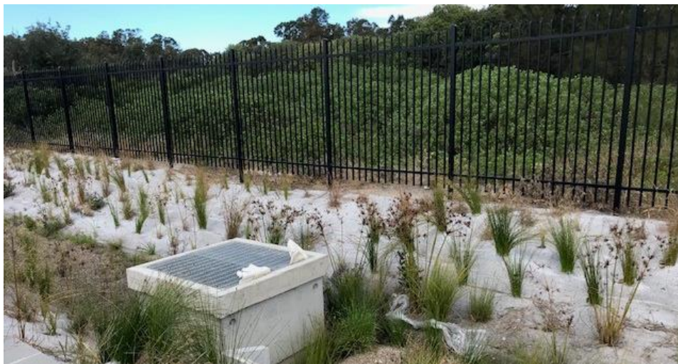
Photo 15 – Stormwater overflow system in place with permanent fencing
