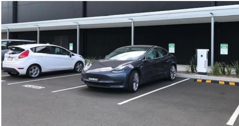
Photo 19 – Electric car charging bays installed and operational
